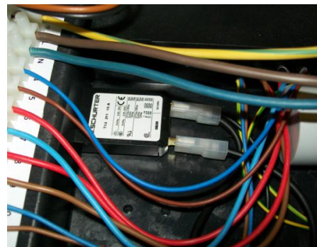
O.T.S. internal control box position
